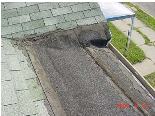
Photo 8 – Flashing and seams are high maintenance.
