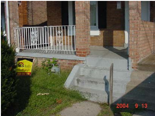
Photo 2 – Railing is loose and improper.
