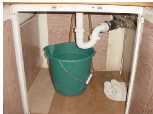
Photo 11 – Buckets and pails are often signs of leaking plumbing.
