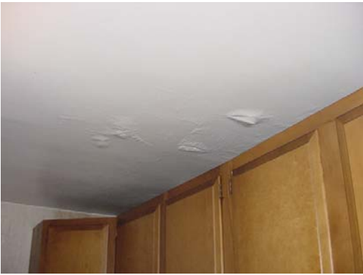
Photo 13 – Peeling paint indicates possible leaks.
